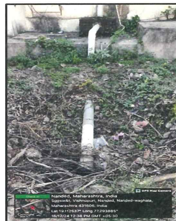
Rainwater harvesting system observed in the campus
