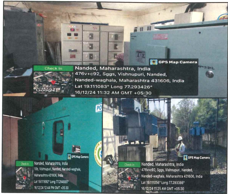
Energy conservation facilities observed in the Campus
